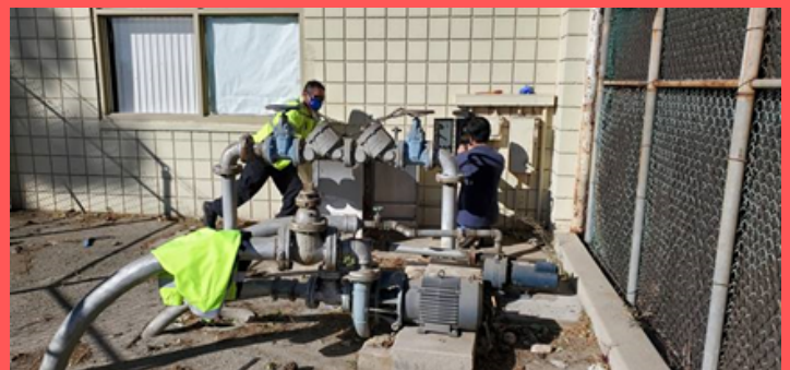
Staff is working on replacing a motor starter and wiring for an irrigation booster pump at Delmann Heights Park
